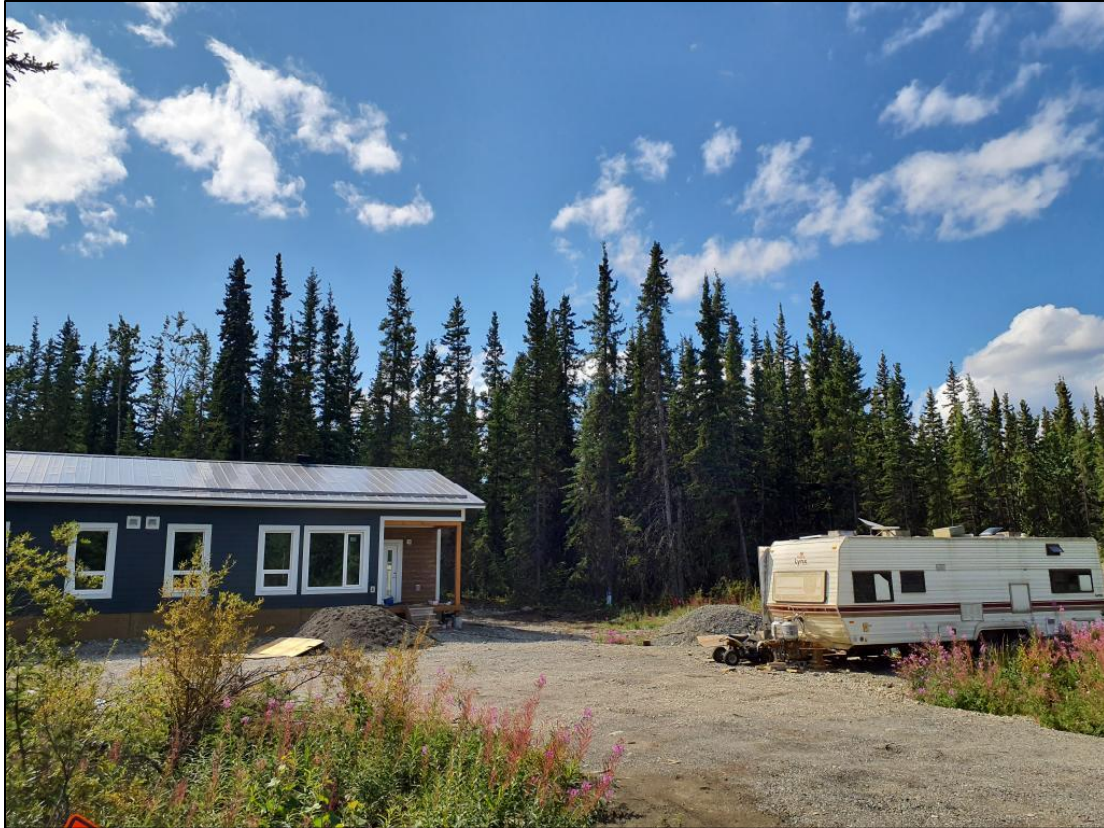
Figure 9: Construction of a new multiplex in the Milk Creek / Squanga subdivision. The structure is very FireSmart though there is untreated and high hazard forest immediately adjacent.
