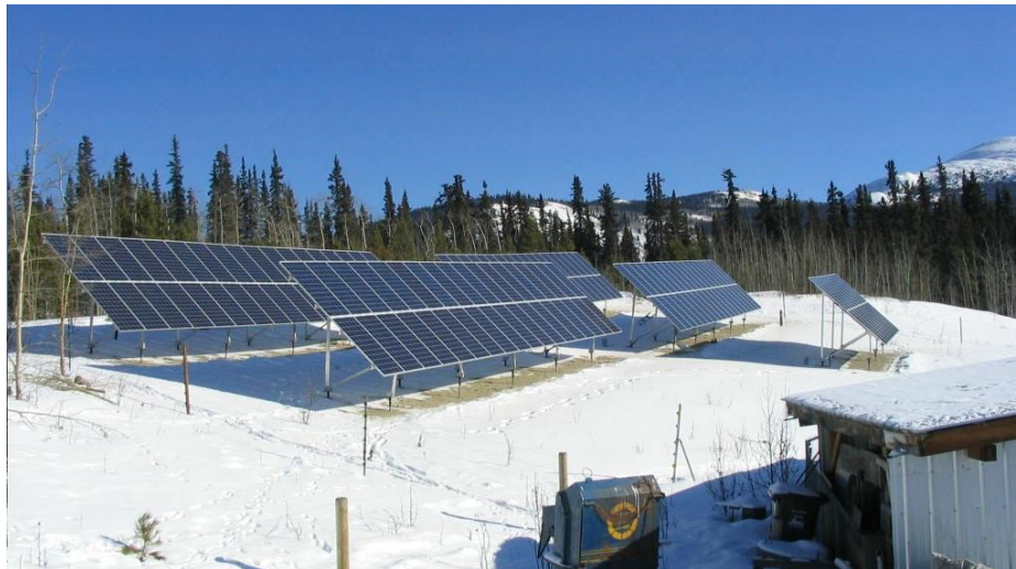
Figure 1 : Mt. Lorne PV array [photo credit: Total North Communications]
