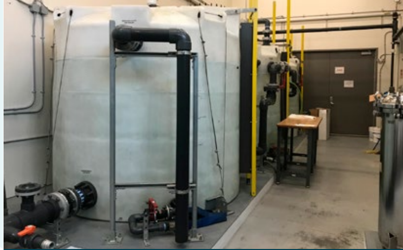
Government of Yukon water treatment plant
