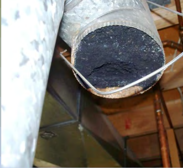
Blocked flue pipe
