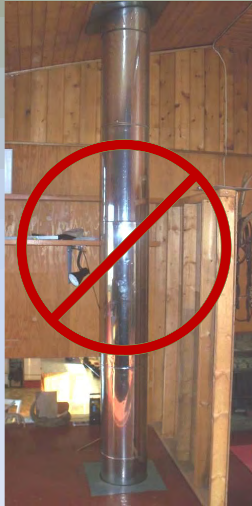
Not enclosed - Non-compliant
