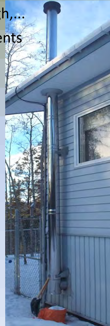
Support Braces & Fire Stop
