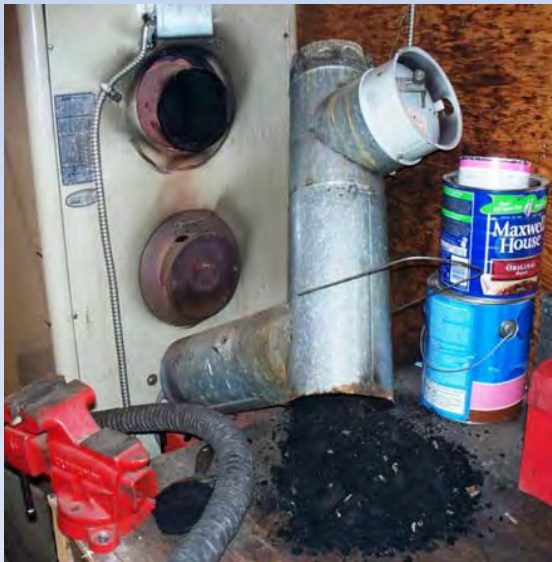
Oil furnace blocked with soot
