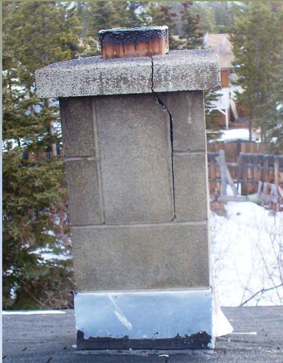
Cracked liner and outer shell - Lost its structural integrity
