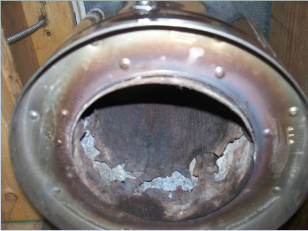
Chimney without a rain cap - Rusted
