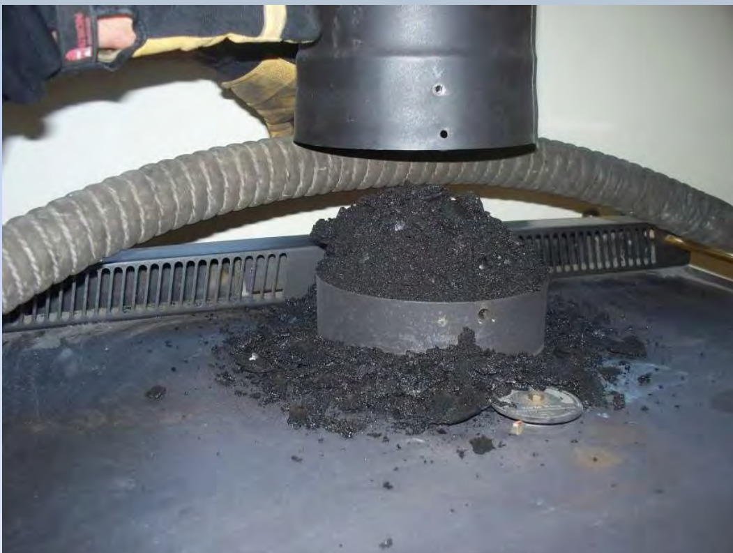
Chimney not swept by a professional
