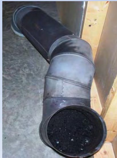
Flue pipe blocked with soot
