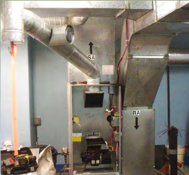
Forced Air Oil Furnace
