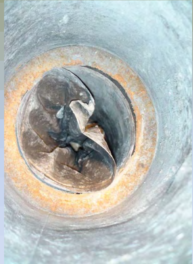
Chimney without a rain cap – Inside liner twisted closed
