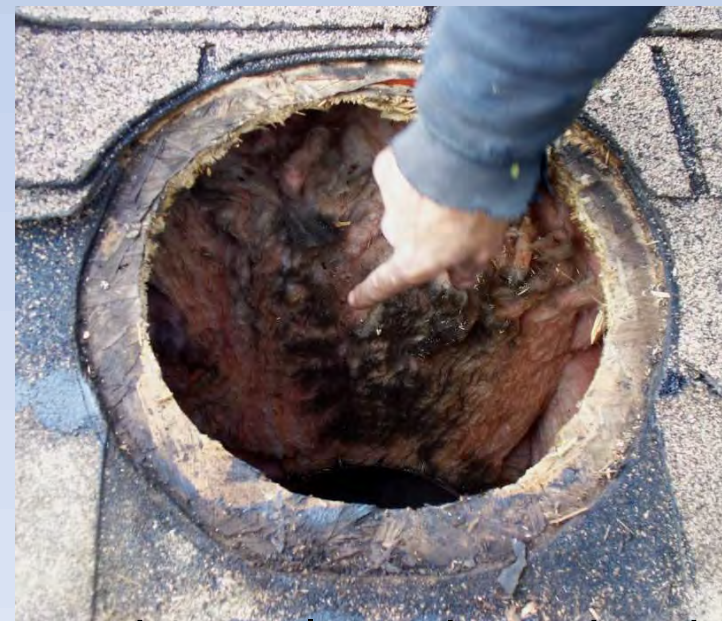
Wood & insulation heated and blackened by heat from chimney
