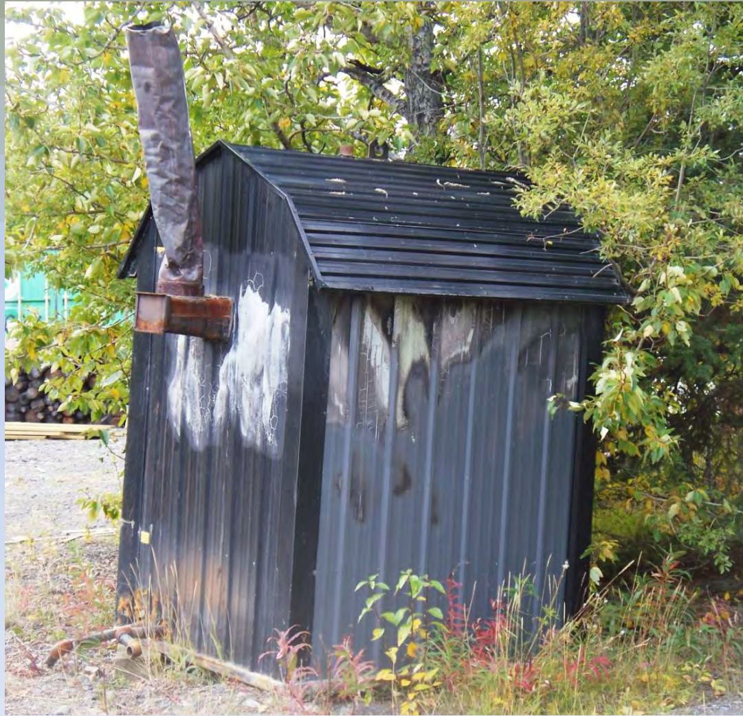
Outside wood boiler destroyed by fire
