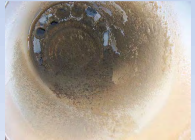
Heat exchanger Waste Oil Furnace
