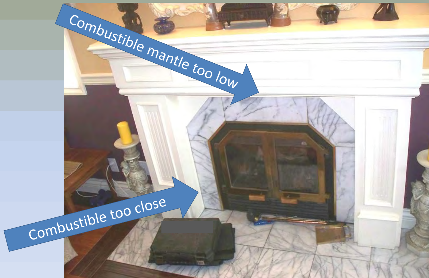
Non-compliant installation - Clearances
