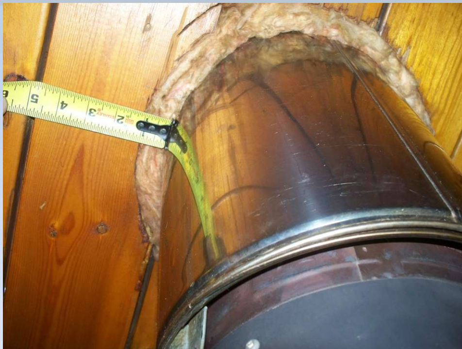
Non-compliant clearances & insulation in contact with chimney
