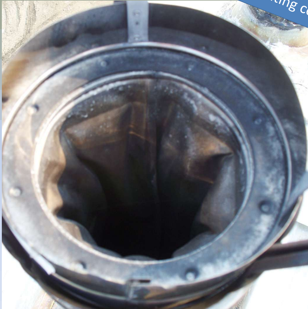
Inside view of chimney used without a rain cap - Buckled
