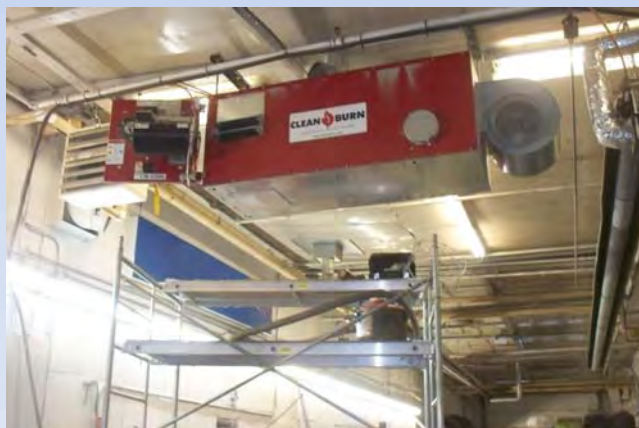
Waste Oil Furnace
