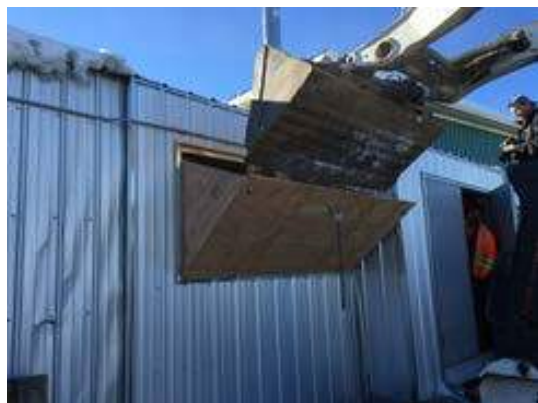
Figure 2-9 - Raven Recycling Biomass System
