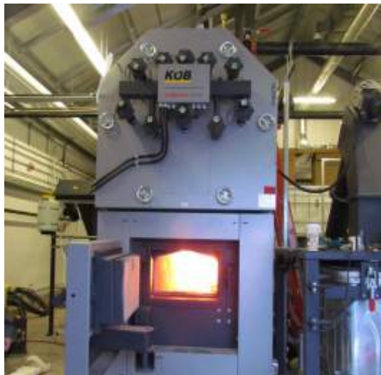
Figure 2-6 - Dawson District Biomass System
