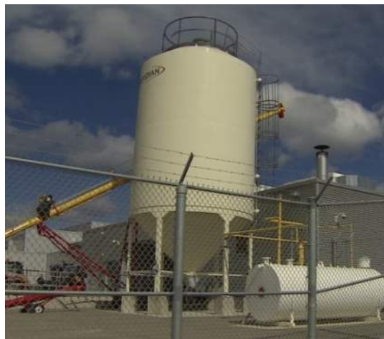
Figure 2-8 - Whitehorse Correction Centre Biomass Boiler
