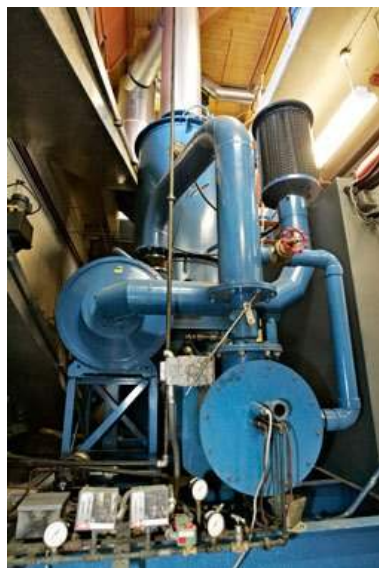
Figure 2-4 - Yukon College Biomass System
