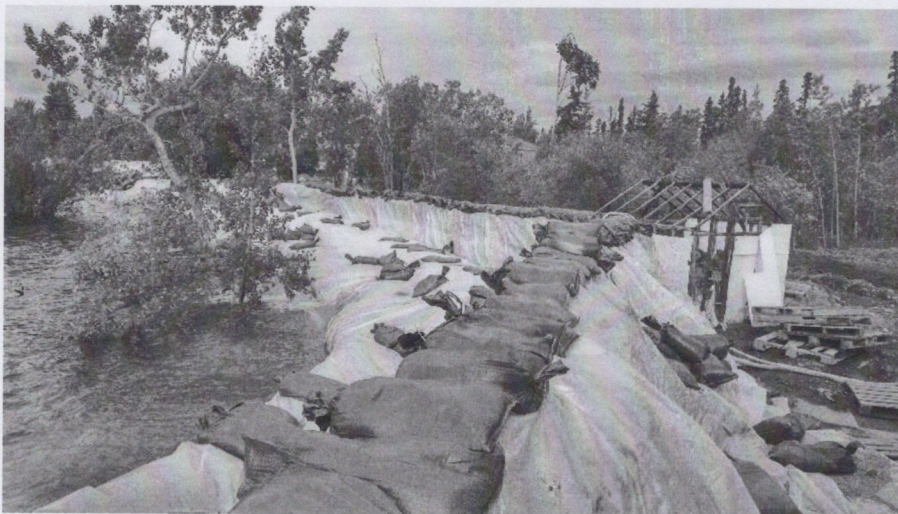
Photo 7. Second Line of Sandbag Dikes Constructed Behind Original Dike Line
