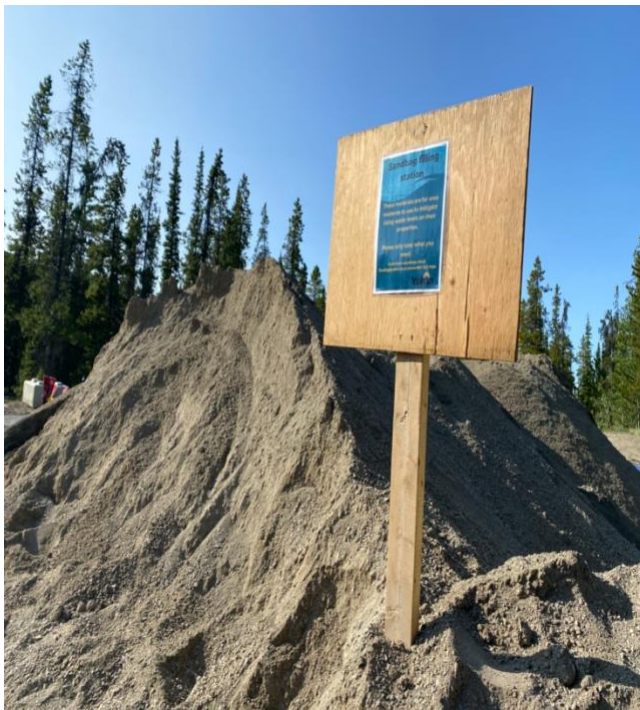
Photo 4: Sandbag filling stations were set up for residents and volunteers to support efforts.
