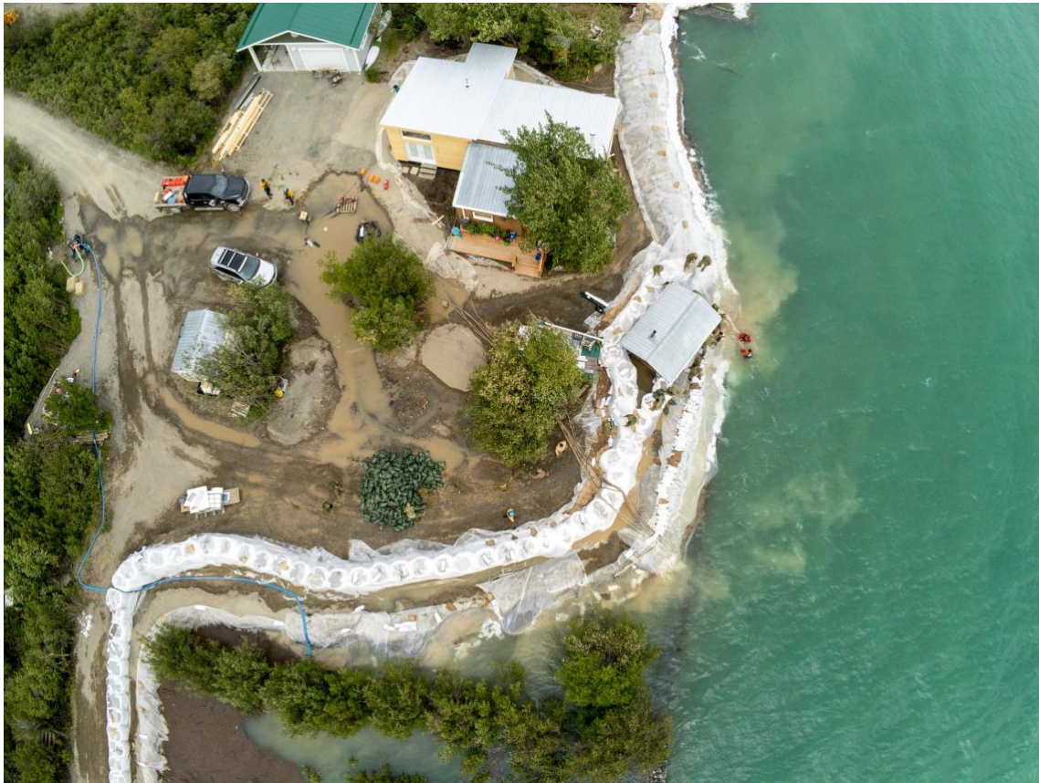
Photo 2 : Members of the Canadian Armed Forces were instrumental to protection efforts at Marsh Lake and Lake Laberge. Here they bolster flood protection infrastructure at Marsh Lake. (Photo courtesy of Government of Yukon)
