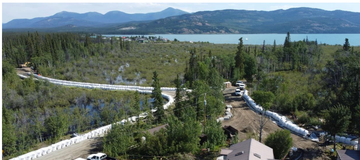
Photo 1: Flood protection infrastructure was constructed to protect access routes and properties at Marsh Lake. (Photo Courtesy: Government of Yukon and Canadian Armed Forces)
