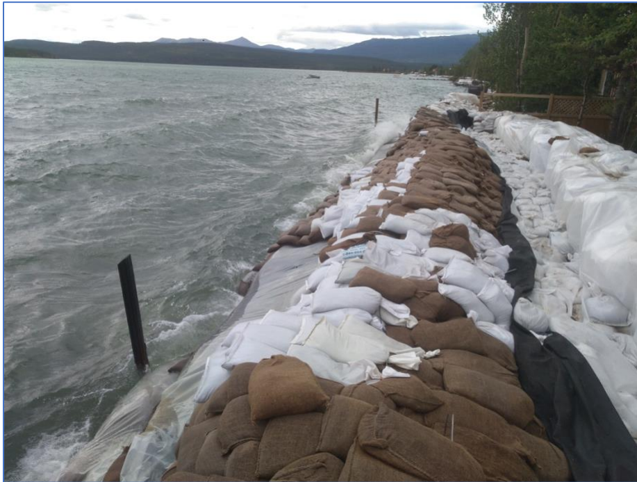
Sandbag berm at Marsh Lake (Photo Courtesy Government of Yukon)
