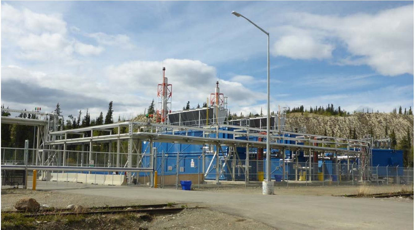
YEC's Liquified Natural Gas (LNG) electrical generating plant
