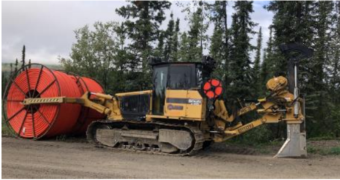
Plow Cat on the Dempster Highway. This machine buries the conduit in the ground.
