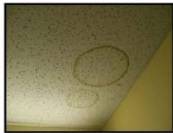
Water-Stained Ceiling Tile
