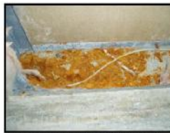
Water-Damaged (Rusted) Metal Bottom Plate
